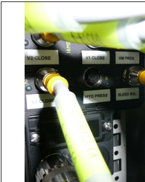
Figure 3 - Hydraulic Pressure Calibration Point
